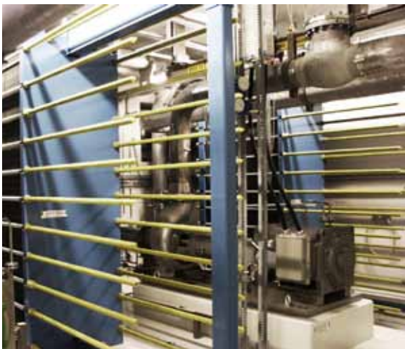
Figure 2: New heat exchangers between the secondary and tertiary cooling circuits.
