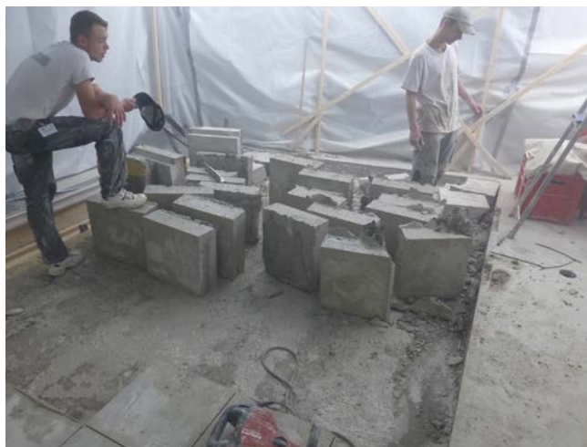
Figure 12: Removal of the old concrete floor inside a dust cover to protect the vicinal instruments from dust released during the concreting work.
