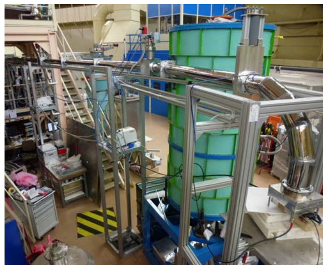
Figure 25: FRM II UCN guide system installed at the UCN turbine exit "testbeam" (on the left, not visible in the picture). More than half of the 17 m long glass guide coated with NiMo was mounted 3.5 m above the floor. UCN traveling from the turbine exit through the guide are detected by a ^{10}\text{B} coated CascadeU detector at the end of the guide (lower right corner).
