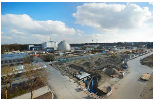
Figure 2: Construction project "Neue Mitte Garching" also poses a challenge to the FRM II.
